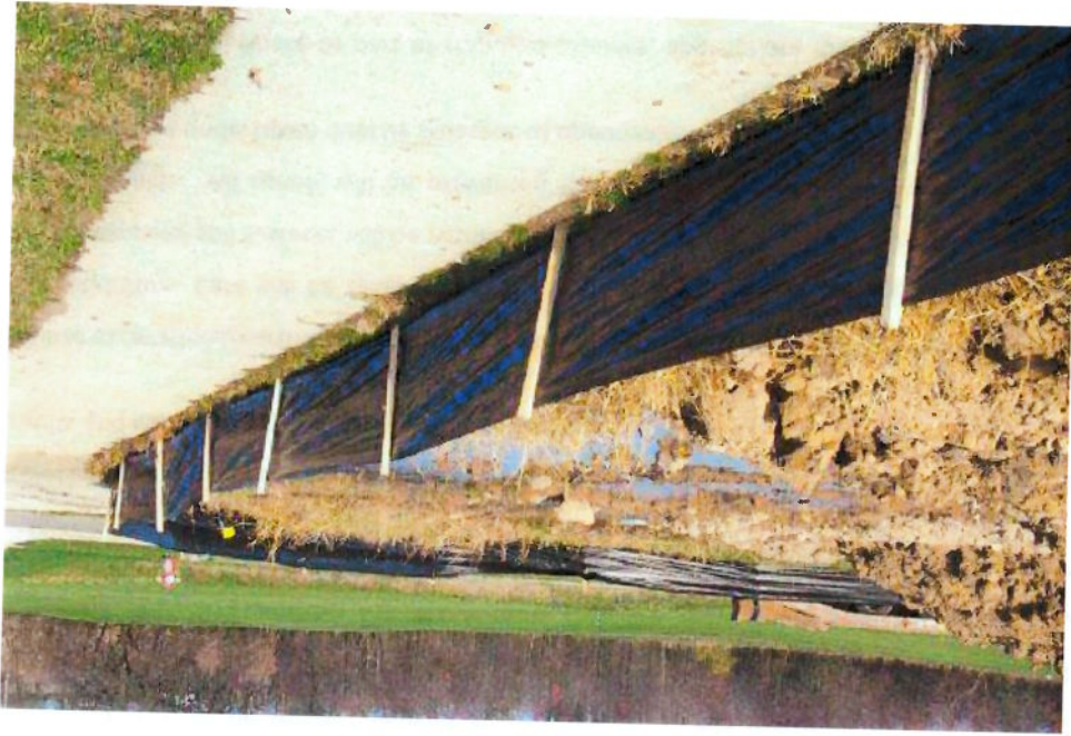
Typical silt fence to be employed
